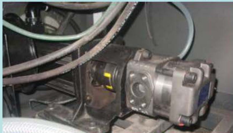
Afterward--- Servo Hydraulic system
